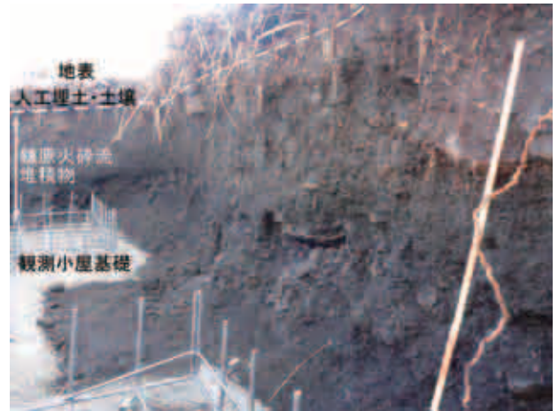
写真2 観測小屋工事現場に露出した鎌原火砕流堆積物 Photo 2 The vertical section of Kambara pyroclastic flow deposit in construction site of observation room.
