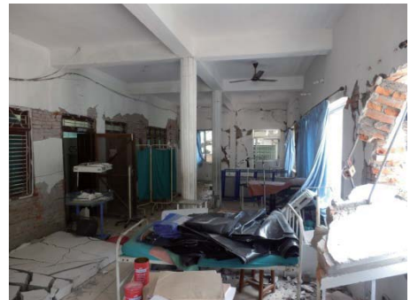
写真 20 病院の被災状況(室内) Photo 20 Damage of the hospital in Khadichaur.
