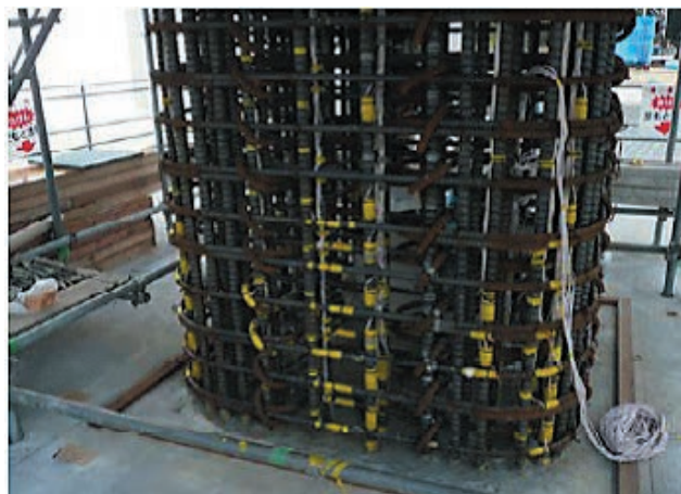
写真 5.3 ひずみゲージの添付 Photo 5.3 Setting of strain gauges prior to pouring of PFRC in column.
