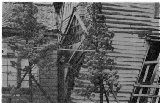
写真—10 建物接続部の被害，柱の座屈もみえる （新潟鉄道教習所・下所島） Damage to the joints between the structures of different story, the buckling of posts also being seen.
