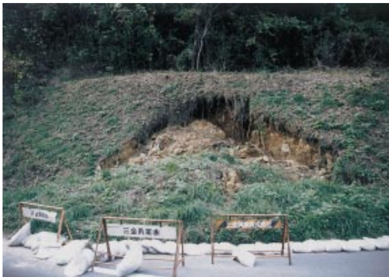
写真19 道路脇の盛土斜面中に生じた崩壊 Photo 19 Landslide on artificial slope of roadside.
