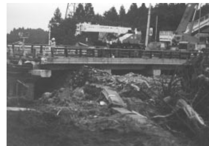
写真4.3 余笹橋の土砂堆積による閉塞状況 [栃木県提供] Photo 4.3 Yosasagawa bridge blocked by sediment.
