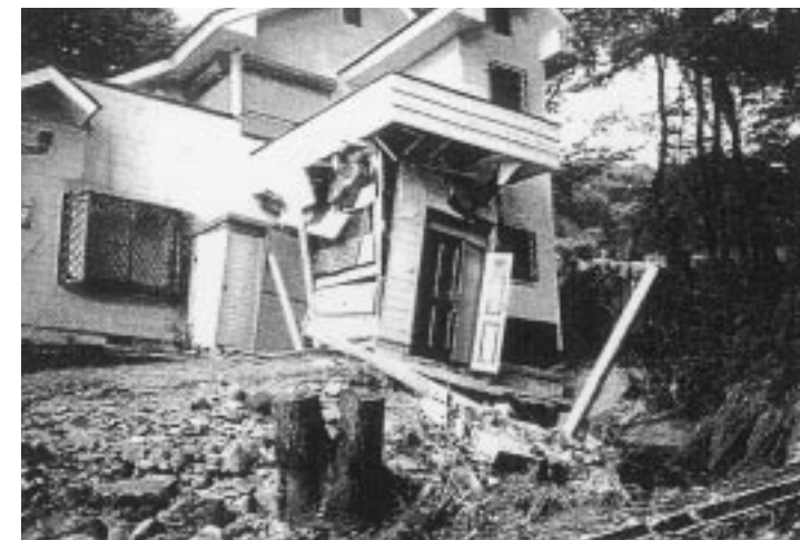
写真2.3 多羅沢川沿いの別荘地被害状況：洪水流の直撃により損壊した別荘 (T3地点) [栃木県提供] Photo 2.3 Resort villa destroyed by flood flow in the valley plain along the Tarasawagawa river : site T3.
