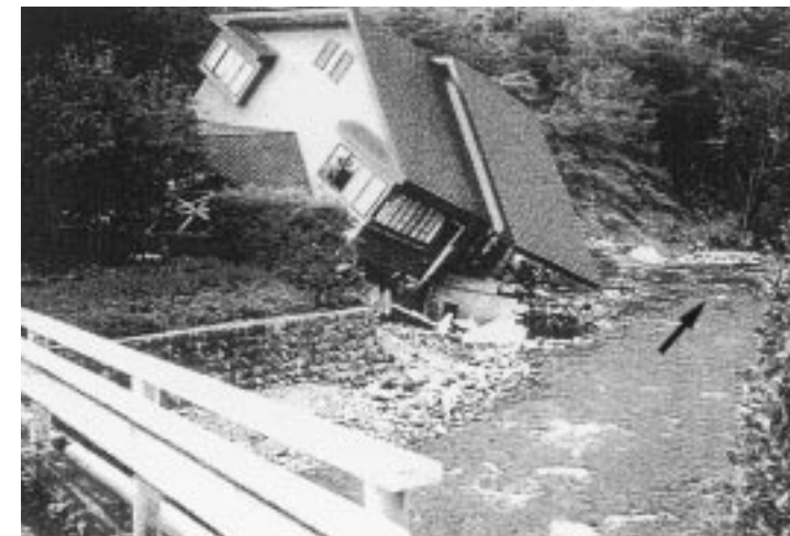
写真2.2 多羅沢川沿いの別荘地被害状況：洪水流の直撃により損壊した別荘 (T2地点) [栃木県提供] Photo 2.2 Damedged resort villa due to the erosion of the river bank and a cottage lot : site T2.
