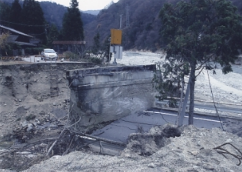
写真 13a 平谷川溪岸の被災状況 Photo 13a Erosion disaster along the Hiratani river.
