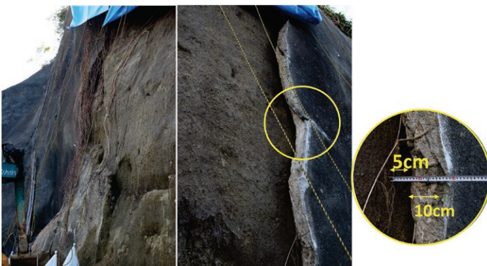
口絵 18 左・右側モルタル切断面と背後地盤との間の状況 Fig. 18 Both sides close up of the mortar sections and rear soils.
