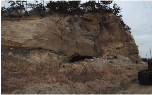
口絵 10 松川浦大橋東側全景(福島県沖の地震で崩壊地点) Fig. 10 Site ①: Full view of East side at the Matsukawaura-Ohhashi point.
