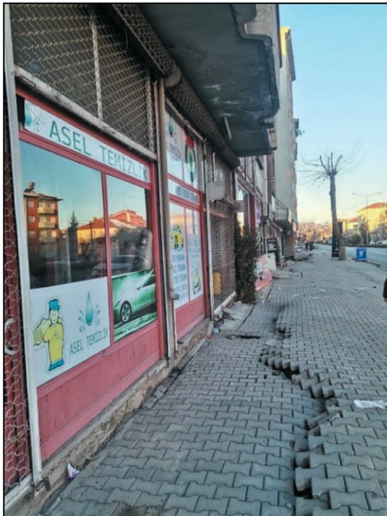
b) Foundation problems in Golbaşı
