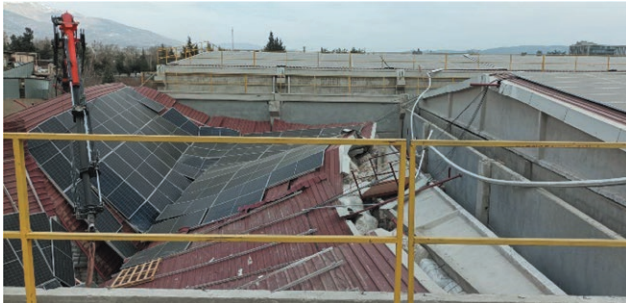
a) Damaged factory roof
