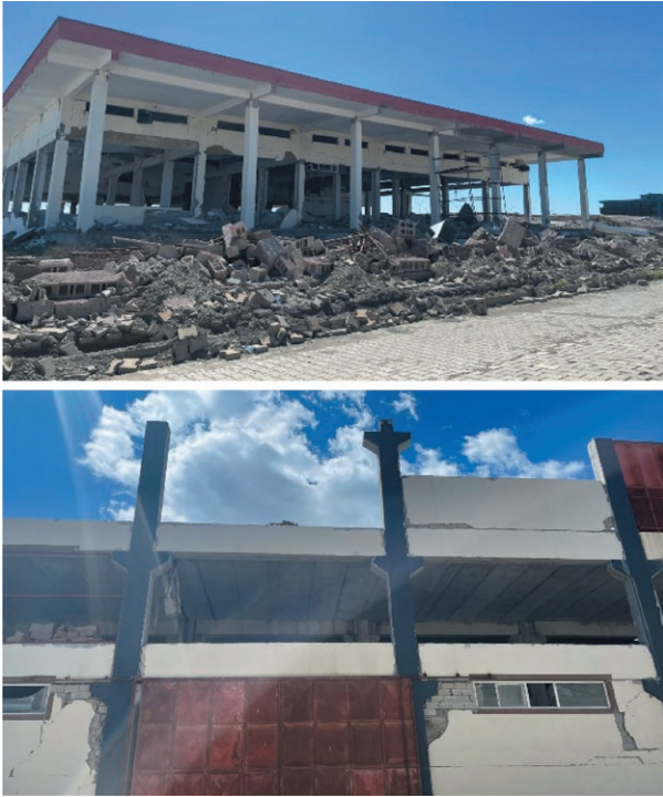
Fig. 3 Structural damage at precast reinforced concrete buildings in Kahramanmaras Turkoglu OIZ due to Kahramanmaras Earthquakes.
