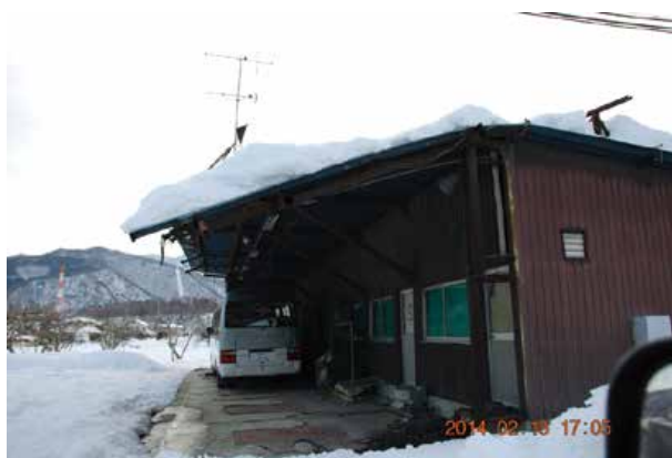
図 24 雪の重みで曲がっている庇(北杜市) Fig. 24 The building which roof bent downward because of excessive snow load (Hokuto City).
