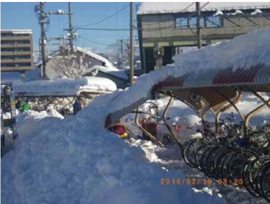
図6 南松本駅駐輪場の屋根の倒壊の様子 Fig. 6 The roof of the bicycle parked by the weight of the snow collapsed (Minami Matsumoto station).
