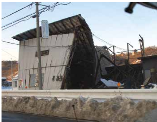
図 23 雪の重みで倒壊した建物(北杜市) Fig. 23 The building which collapsed because of excessive snow load (Hokuto City).
