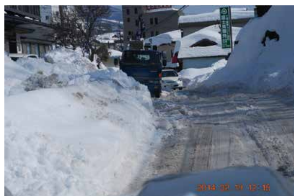
図22 除雪作業中の生活道路(富士見駅付近) Fig. 22 Community road during snow removal operation near Fujimi Station.
