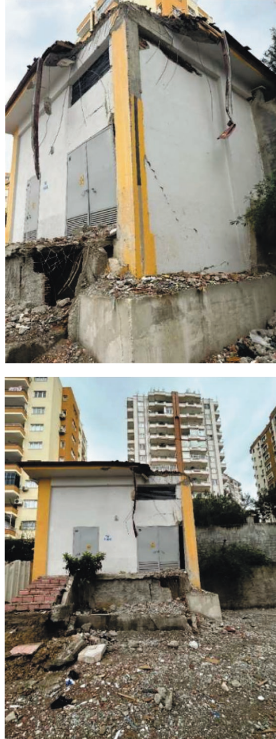
Fig. 2 Adana City Transformer Center TR184 Damage 17) .
