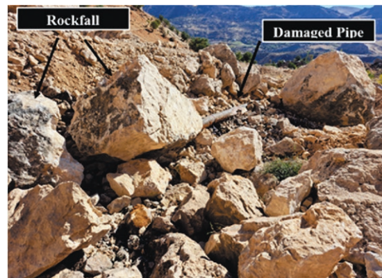
Fig. 6 Pipe Damages at Gurlevik Spring, Adiyaman 2) .
