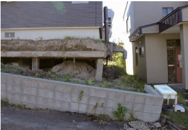
図12 札幌市清田区の液状化(杭基礎)(撮影日9/17) Fig. 12 Liquefaction of Kiyota-ku, Sapporo (Pile foundation) (shooting date 9/17).
