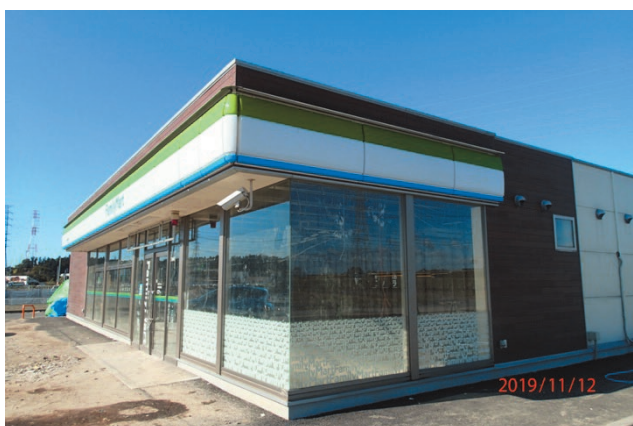
写真2 天井付近まで浸水したコンビニストア(M3) Photo 2 Flood water almost reached the roof of the convenience store at investigation location M3.
