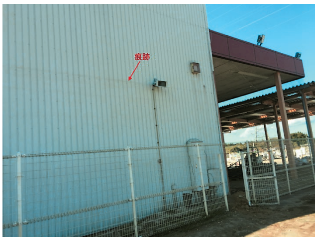
写真3 M6の店舗の外壁に残される浸水痕跡 Photo 3 Water line from flood waters visible on the store wall at investigation location M6.
